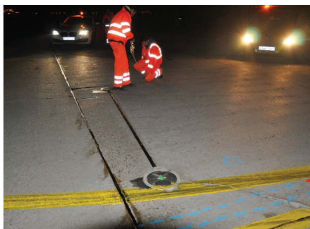
Fig. 5: Damaged concrete slab with two built-in components
