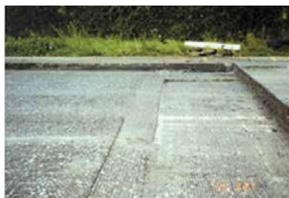
Figure 3: over-thickness building up gradually at the transition between the new concrete and the existing pavement
