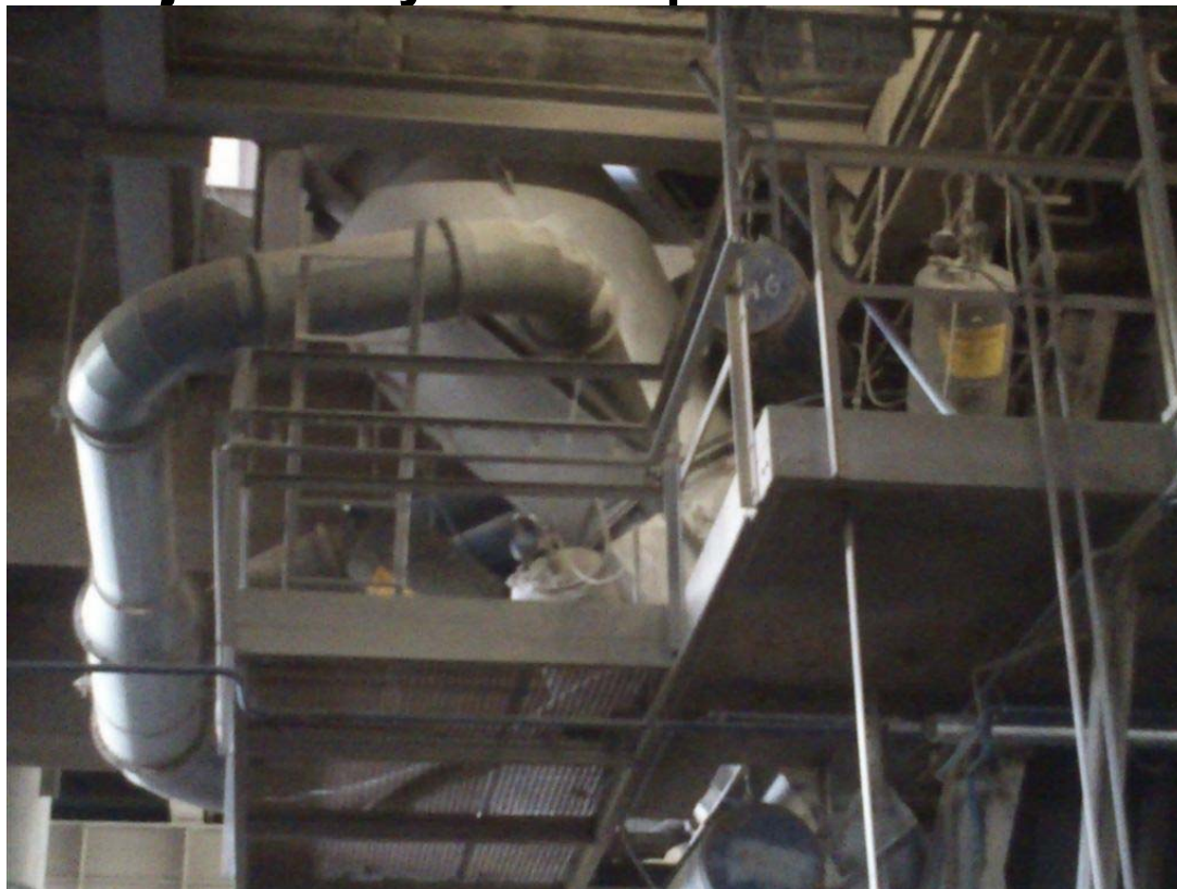
Bypass gases into the cooler – JAN BOHUNEK
