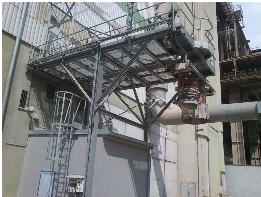
Bypass gases into the cooler – JAN BOHUNEK
